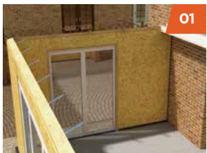
Structural ringbeam is sealed and secured to the top of the wall structure.
