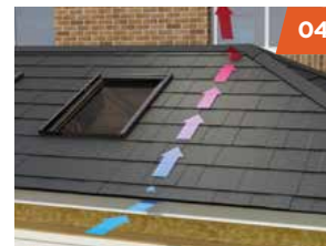
Roof is batted and chosen tile is added ensuring weather-tightness. The gutter and external trim are secured.
