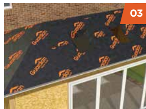
Breathable waterproof membrane is laid over the structural OSB 3 and secured in place.
