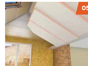
3 layers of high performance insulation (between and over rafters, and insulated plasterboard), is installed.
