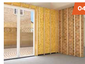
The interior has services added and is batted ready for internal finish.
