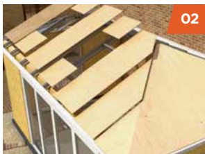
The aluminium roof structure is secured to the ring-beam and structural OSB 3 is fixed.
